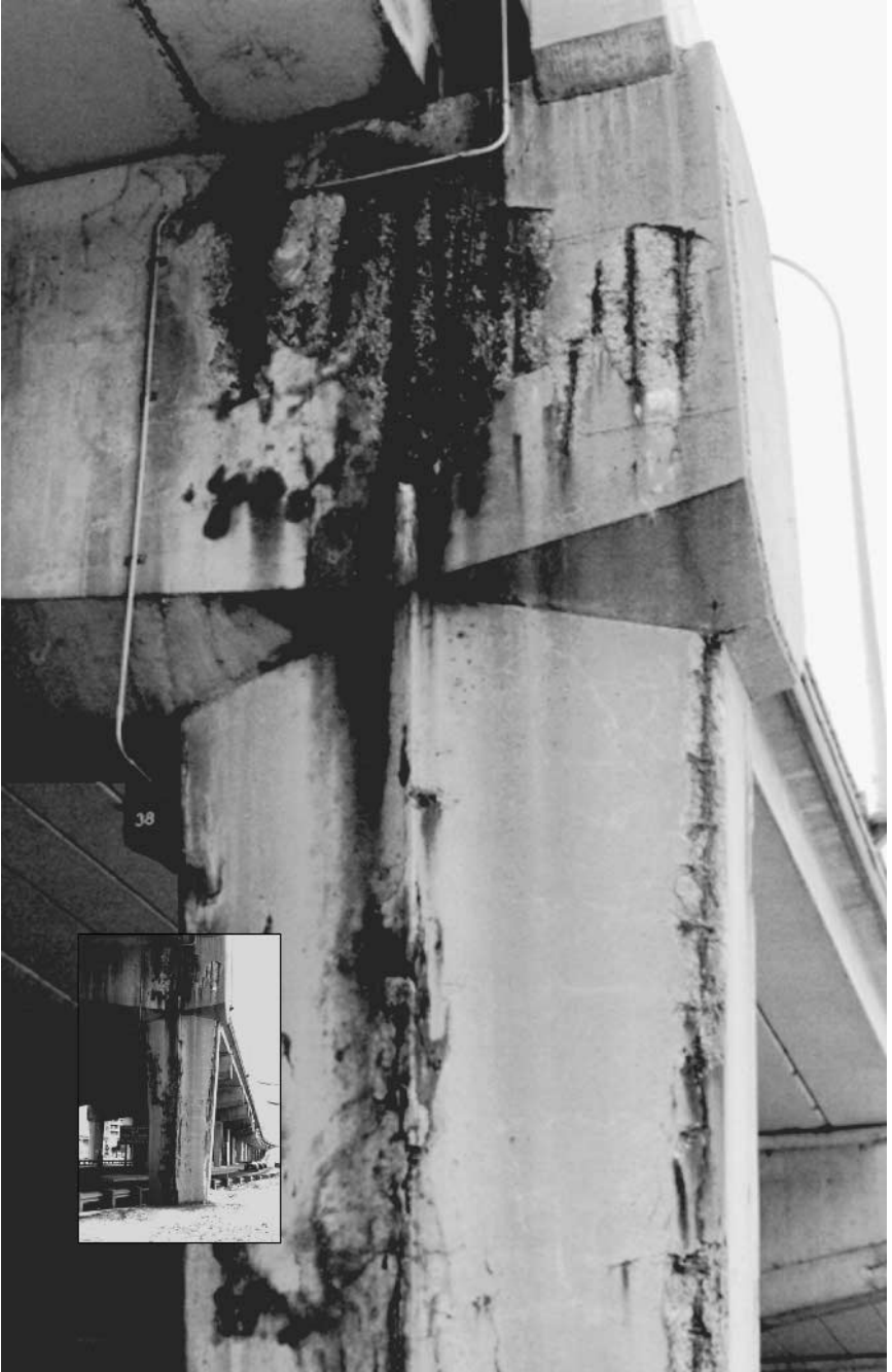
Figure 2.27 Concrete degradation caused by rebar corrosion damage in a highway structure in downtown Toronto, Ontario. Extensive repair work was underway on this structure at the time the picture was taken. The annual maintenance costs for this structure were recently reported at around $18 million.
