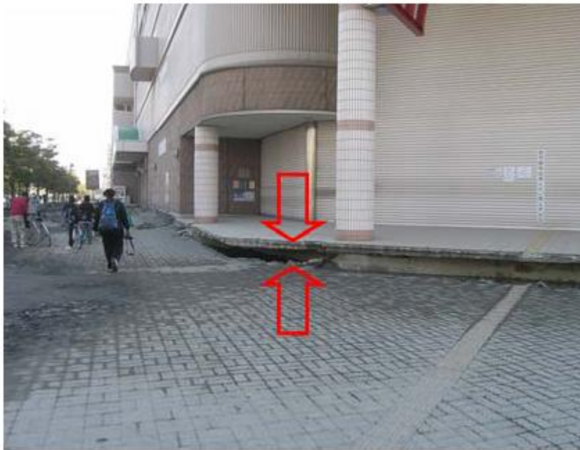
Fig. 15 45-cm subsidence of ground surface in front of a shopping center (Urayasu City)
