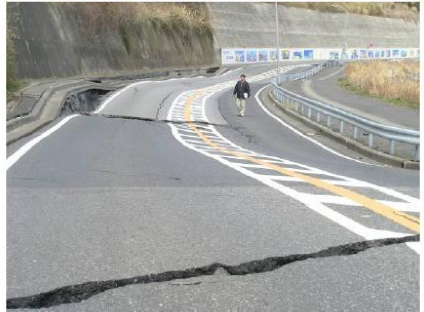
Distortion of road embankment
