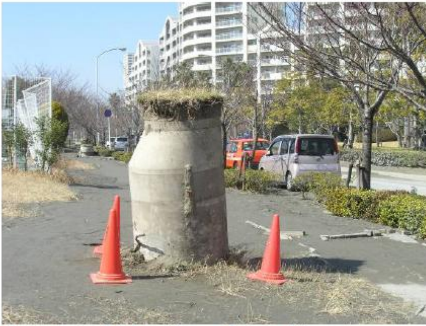
Fig. 18 Uplifting of manhole of 2 meters In Urayasu of Chiba
