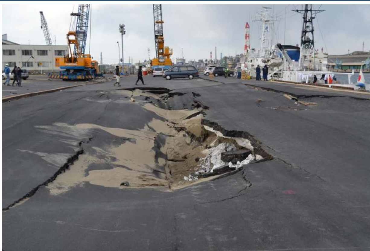
Figure 13a. Depression behind quay wall that displaced towards water at Kashima port (N35.88461, E140.68476).
