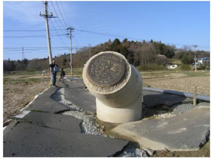
Fig. 19 Uplifting of manhole and surface subsidence in Sukagawa of Fukushima
