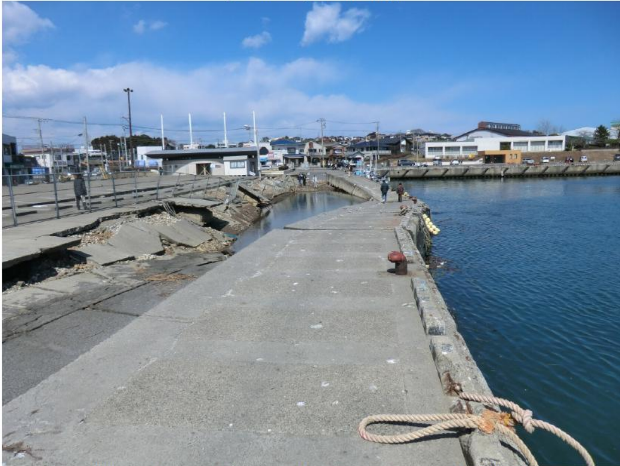
Figure 13b. Displacement of quay wall at Hitachinaka port (N36.341, E140.596).
