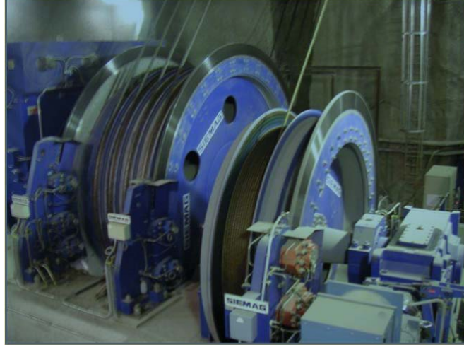
4 Rope Main Cage Winder and Single-Drum Auxiliary Winder
