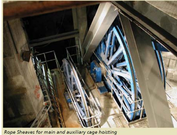
Rope Sheaves for main and auxiliary cage hoisting
