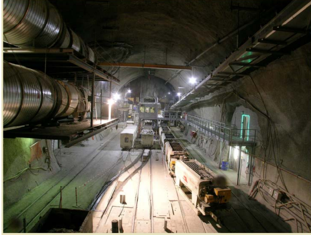
Mine car circulation and decking plant
