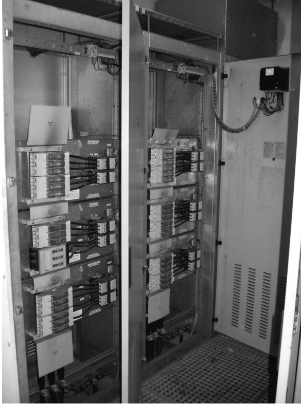
Figure 11.8 Two of five cubicles with total reactive power of 1400 kvar, 400 V, 50 Hz for the purpose of compensating reactive power on the MV side (20 kV) via its own transformer of 1600 kVA (see Figure 11.9). Reproduced by permission of Stahlwerk Annahütte Max Aicher & Co KG, Germany.
