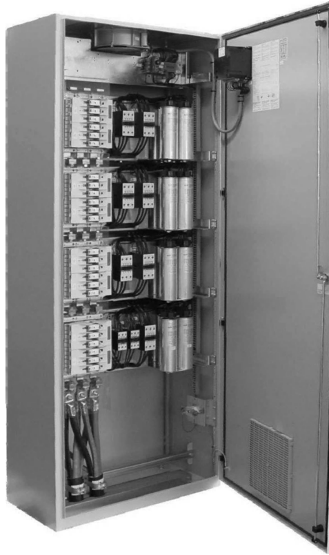
Figure 11.2 Reactor-protected compensation bank of 400 kvar, 400 V, 50 Hz, 16 \times 25 kvar. Reproduced by permission of Frako Kondensatoren und Anlagenbau GmbH, Germany.
