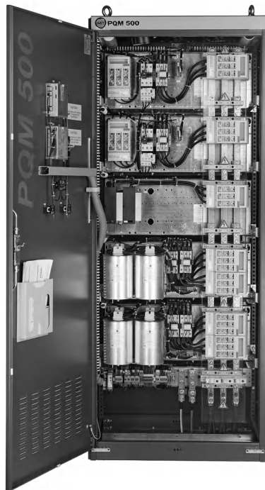
Figure 11.16c Compensation bank combining three technologies of reactive power control via air contactors as well as static contactors and control of passive filters. Reproduced by permission of Maschinenfabrik Reinhausen GmbH, Germany.
