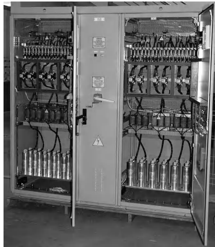
Figure 11.16a Compensation bank of 300 kvar; 440 V, 60 Hz; switching in 12 steps of 25 kvar each; reactor protection p = 7\% . Reproduced by permission of General Motors do Brasil, Brazil.
