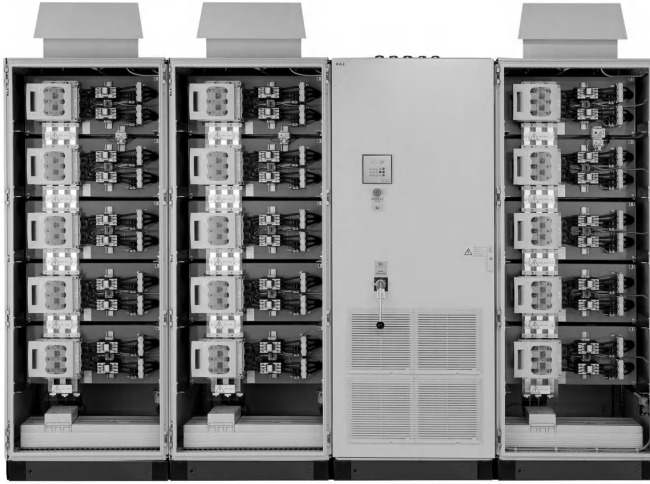
Figure 11.16d Compensation bank of 1500 kvar; 690 V, 60 Hz; reactor protection p = 7\% ; for offshore oil platform. Reproduced by permission of System Electric GmbH, Germany.
