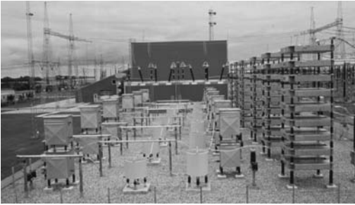
Figure 1 HVDC converter station with ac filters in the foreground and valve hall in the background
