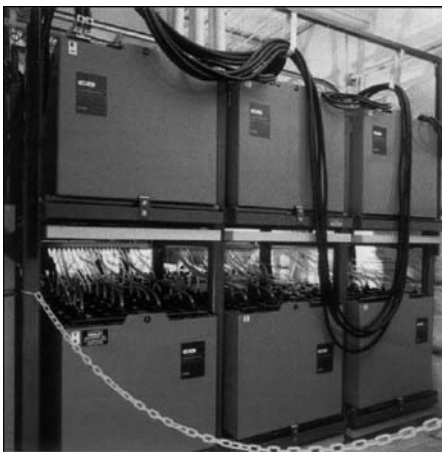
Figure 6 Large lead-acid battery bank
