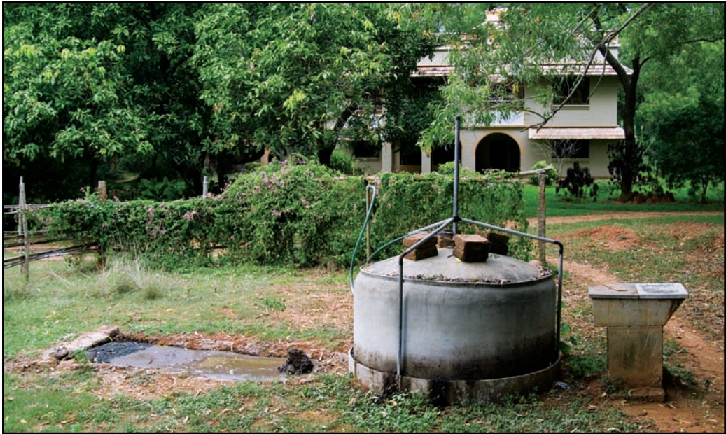
A biogas digester turns animal waste into biogas, which can be used as fuel.
