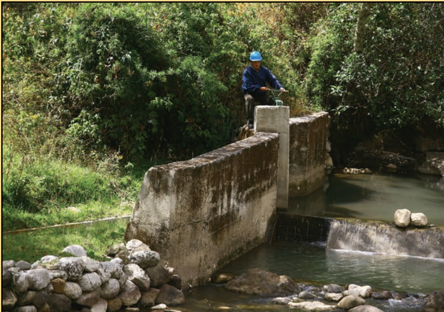
A worker adjusts part of a small hydropower plant in Peru.
