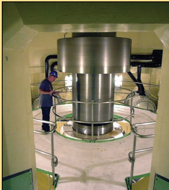
Part of one of the power plants on the Niagara River.
