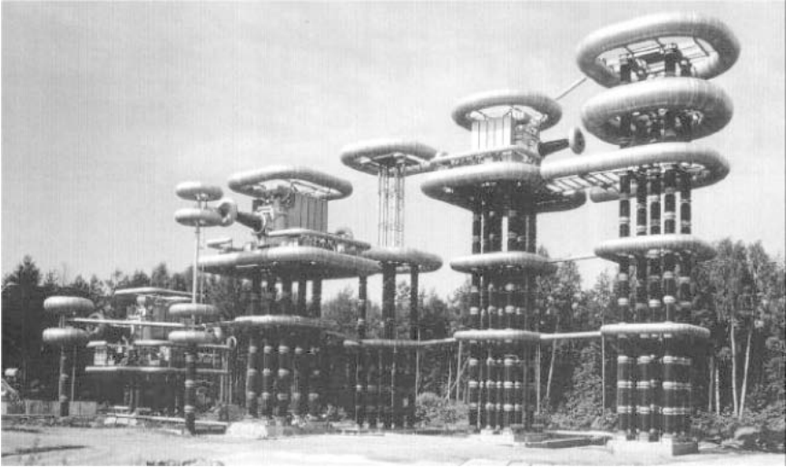
Figure 2.16 (b) Cascaded testing transformers with metal tanks and coolers. Total voltage 3000 kV, 4 A (courtesy HIGH-VOLT Dresden, Germany)
