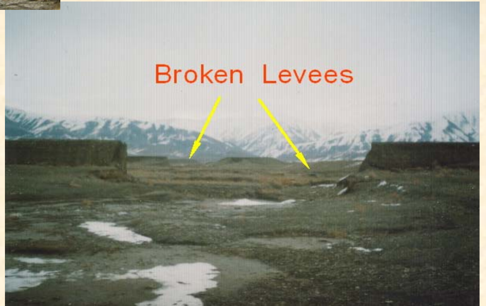
Upstream views of Faroobroman broken cross-levees
