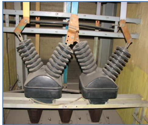
Connection of 2 voltage transformers in V arrangement (does not allow use of neutral voltage displacement protection or residual voltage measurement).
