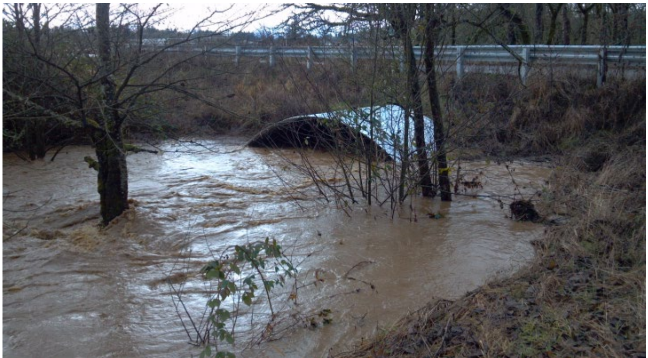
Ineffective flow at the entrance to a culvert
